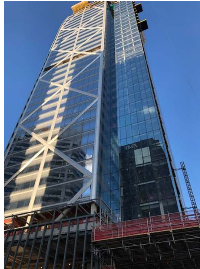
Picture: Project with evguard® laminating film in Downtown tower of commercial bay development, New Zealand.
